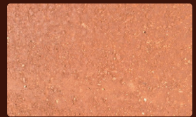
Close-up of the road surface immediately after treatment with OFB Bind and Seal
